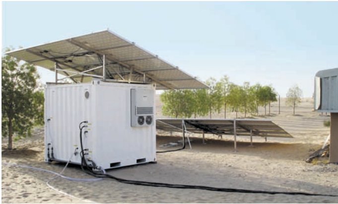
TBC 100: solar powered brackish water container located in the desert, Abu Dhabi 2009
