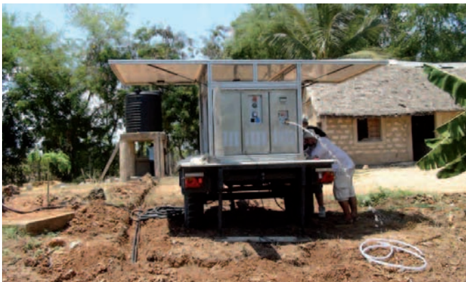
TWS 200: treatment of organically contaminated borehole water in the Children's Village Diani, Kenya 2010
