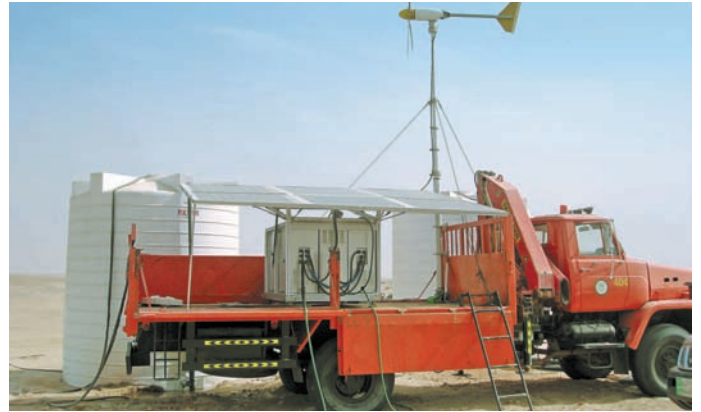
TSS 200: treatment of brackish water incl. wind generator in the desert of Abu Dhabi, 2010
