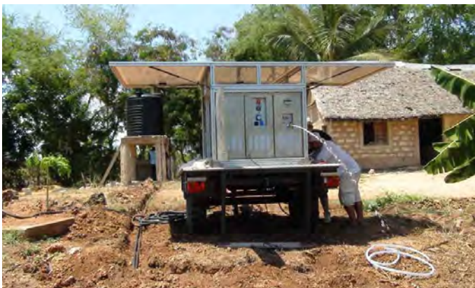
TWS 200: treatment of organically contaminated borehole water in the Children's Village Diani, Kenya 2010
